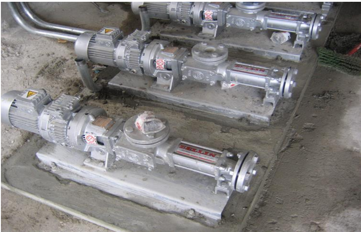
Sludge Pumps General Appearance
