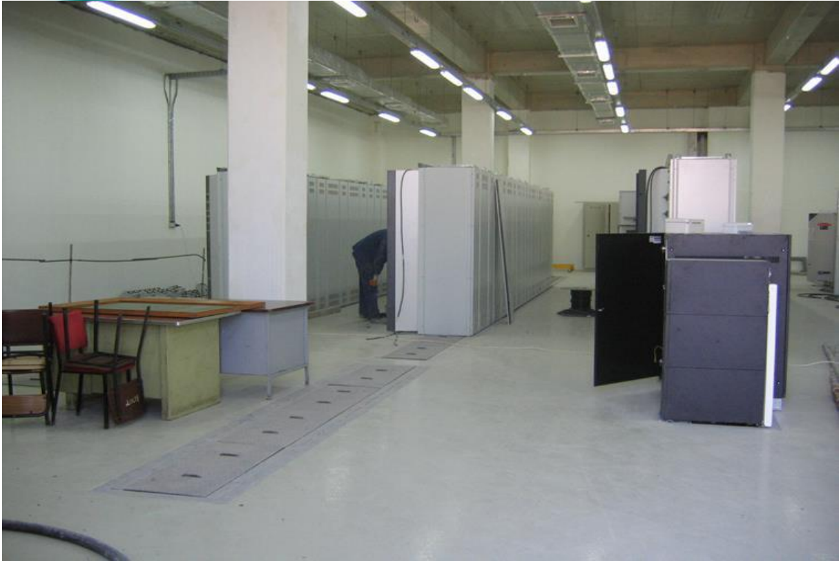
MCC PLC Cabinet General Appearance
