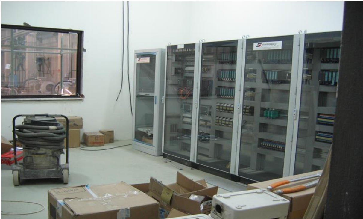
Operator Room and PLC System Cabinet
