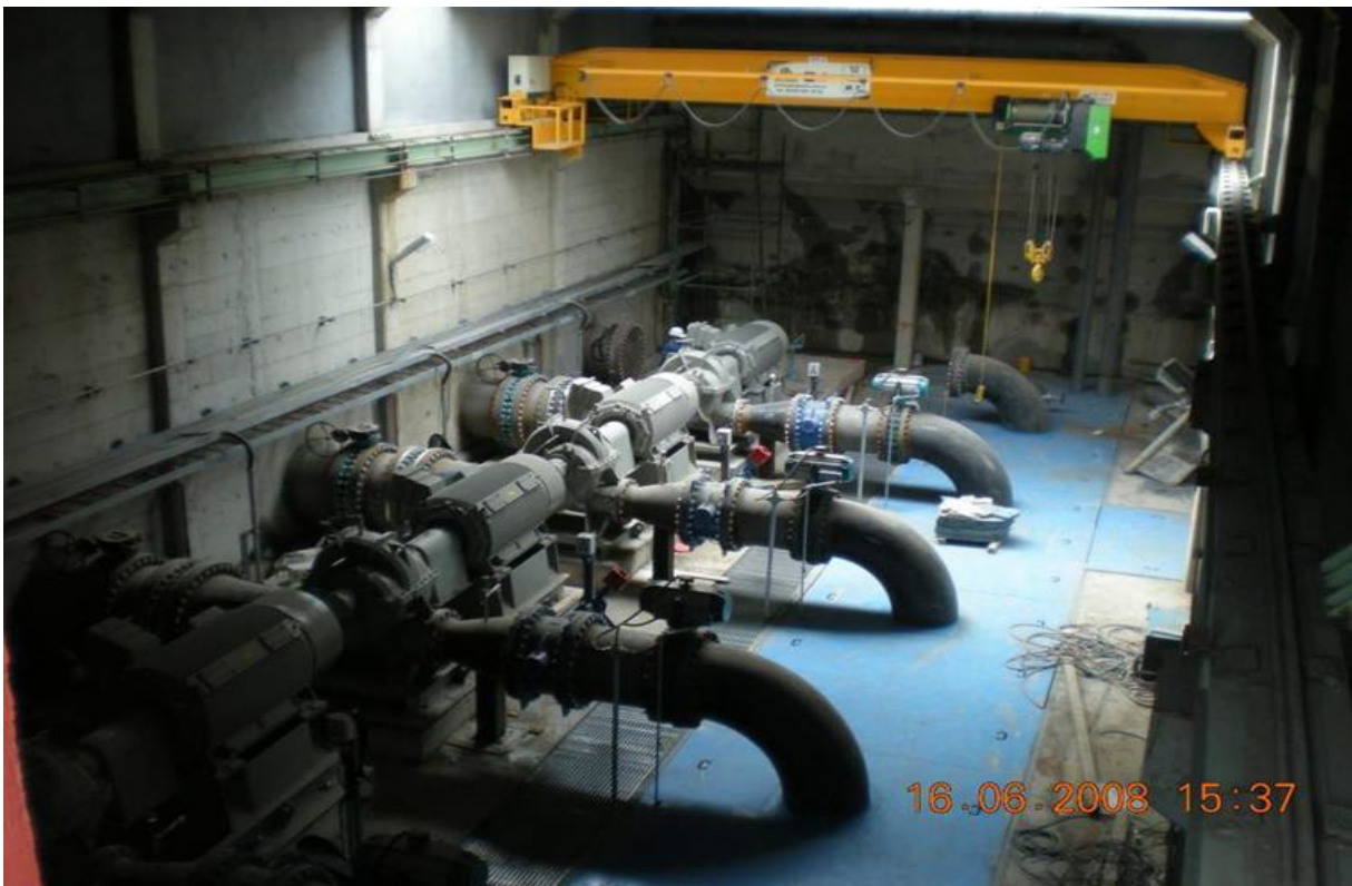
Settling Basin Clean Water Pumps
