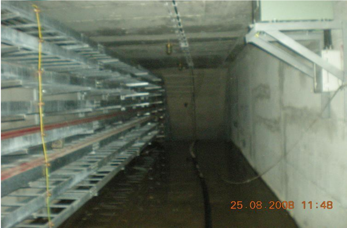
Cable Gallery General Appearance
