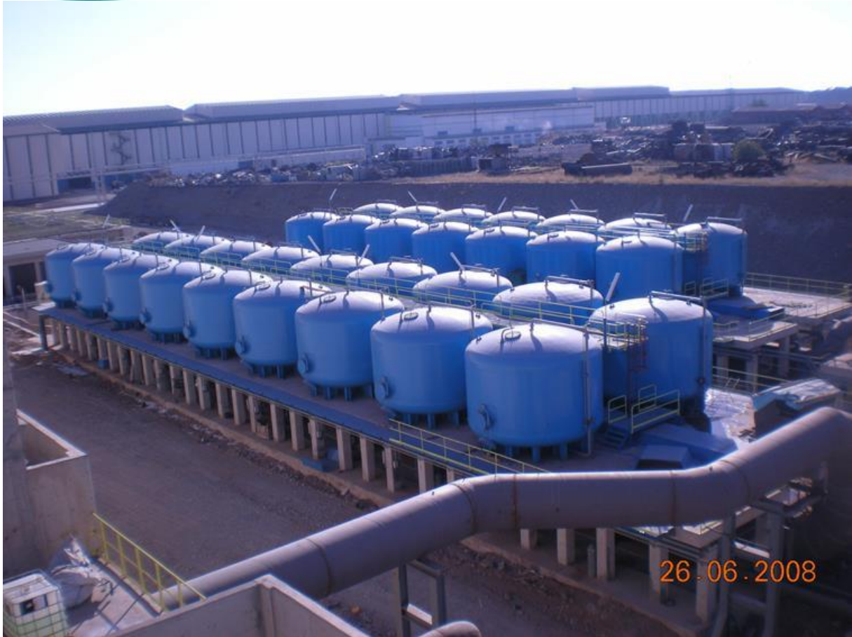
Sand Filter Area General Appearance
