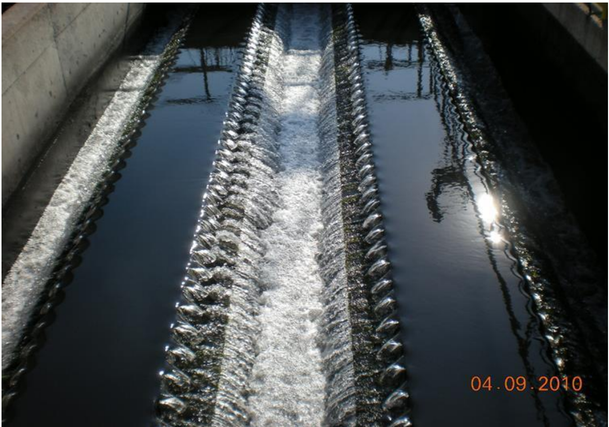
Settling Basin Clean Water
