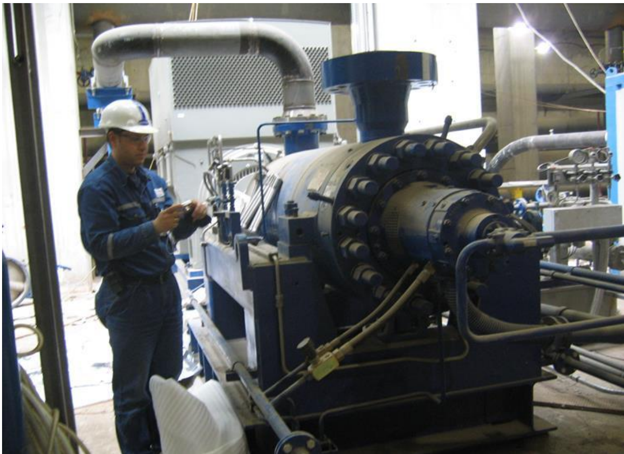
Descale Pump General Appearance
