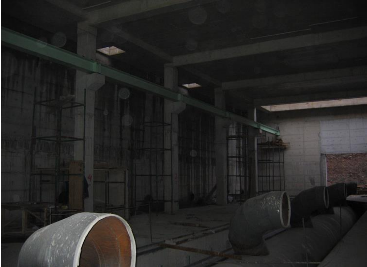
Pump Discharge Hall
