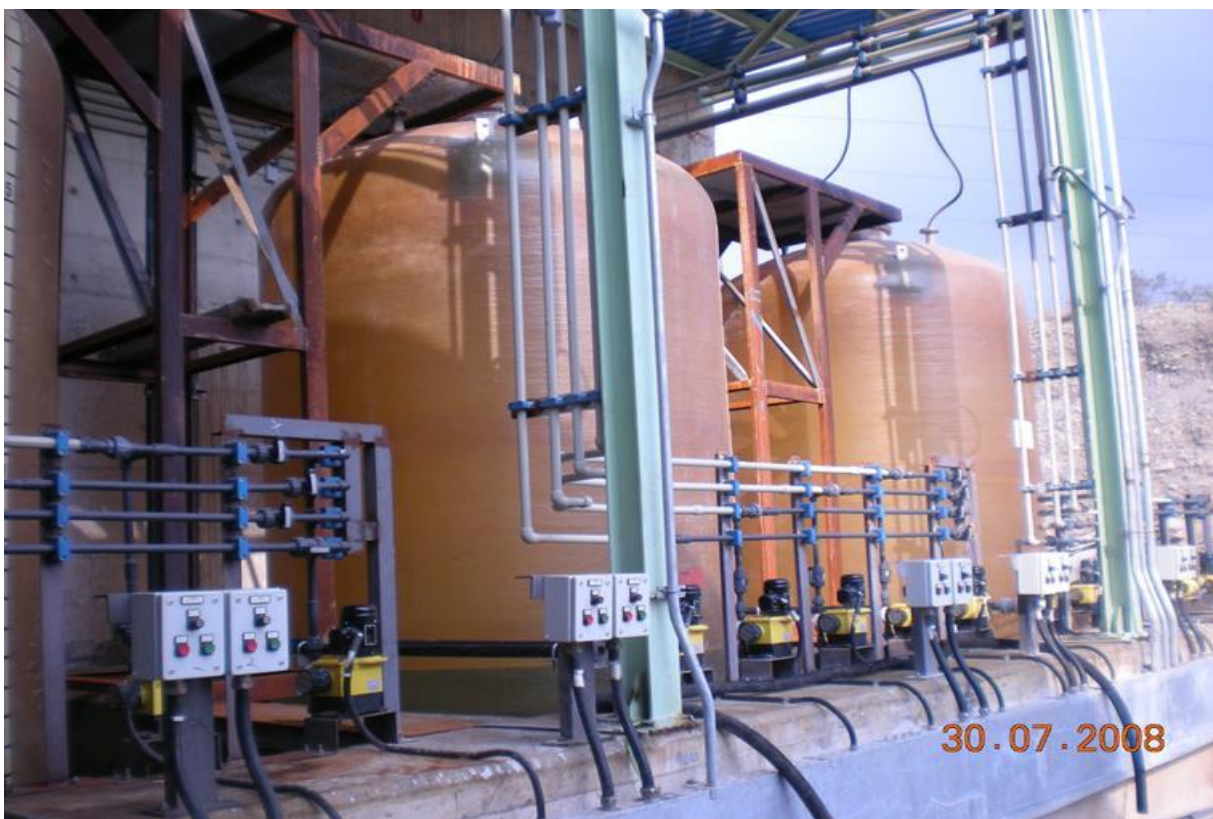
Chemical Dosing Units General Appearance
