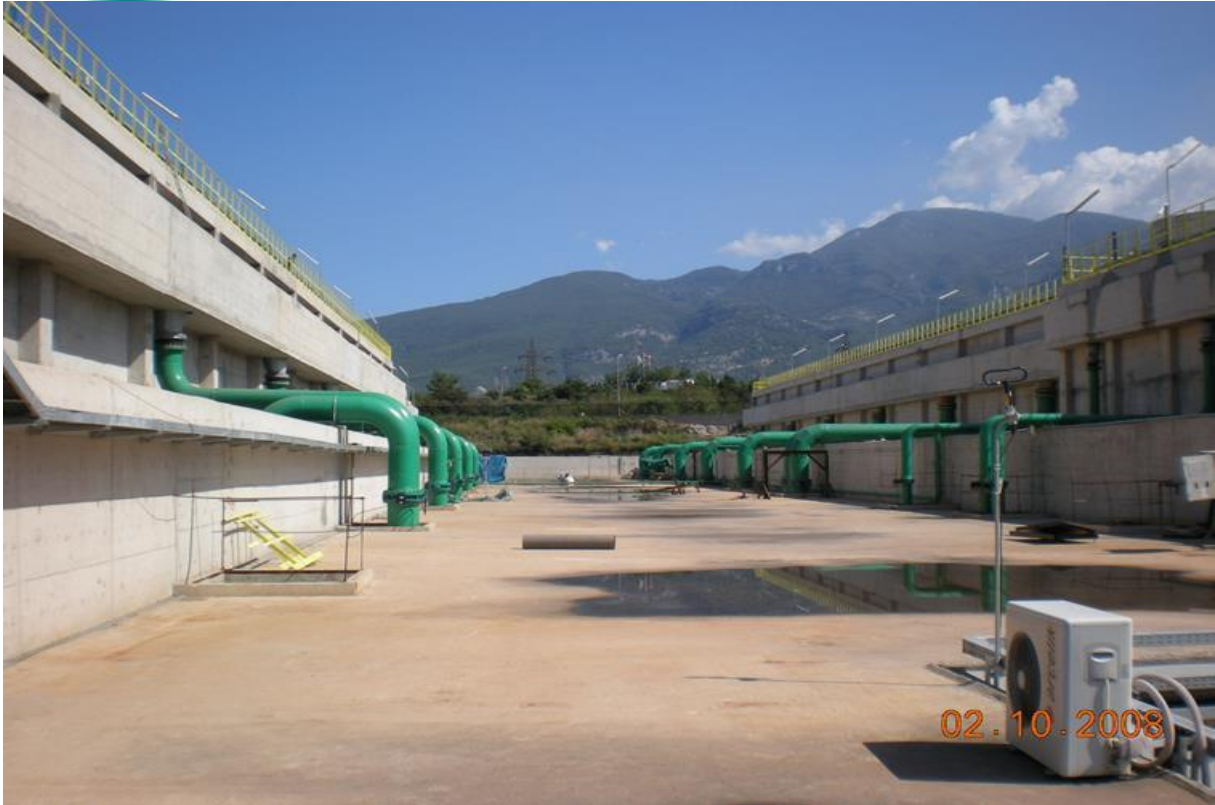
Cooling Towers General Appearance
