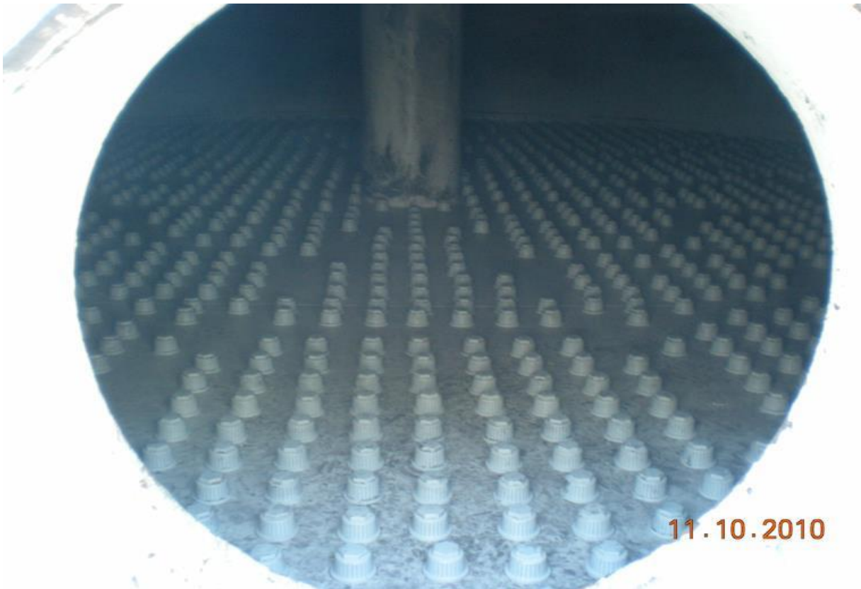
Sand Filter Inside Nozzles Filters
