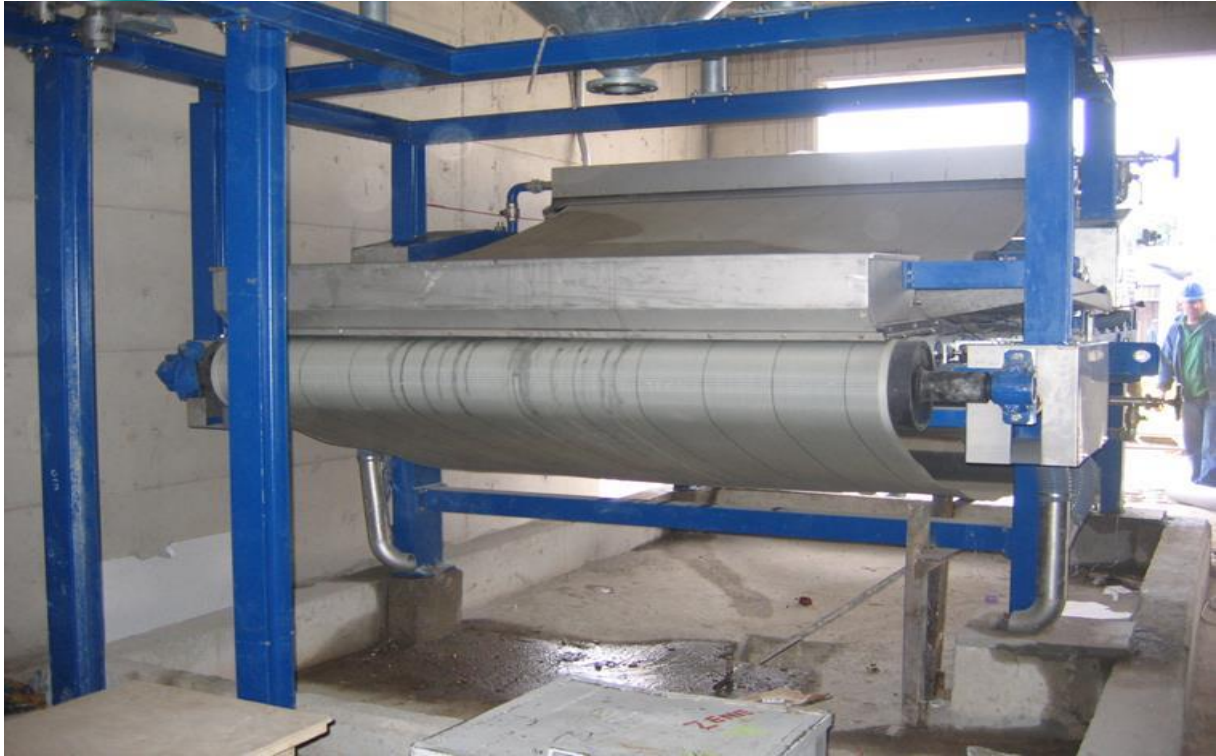
Sludge Belt Press General Appearance
