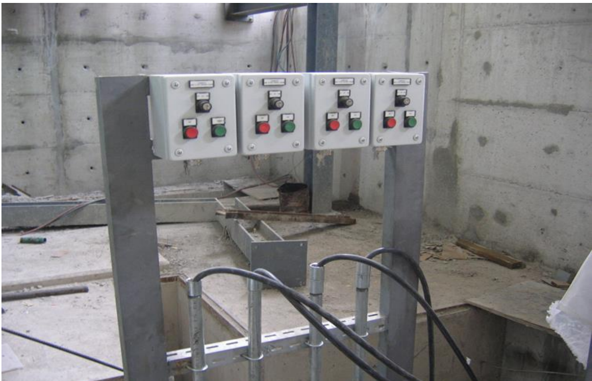
Pump Area Control Box General Appearance
