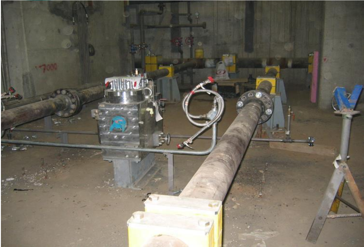
Descale Pump Discharge Line and Valve General Appearance
