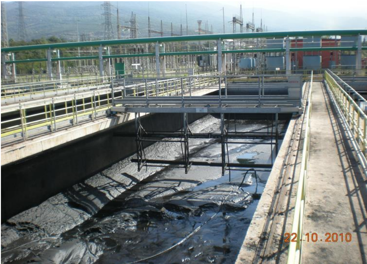
Settling Basin Scraper Bridge
