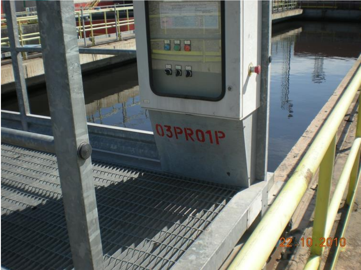
Settling Basin Scraper Bridge
