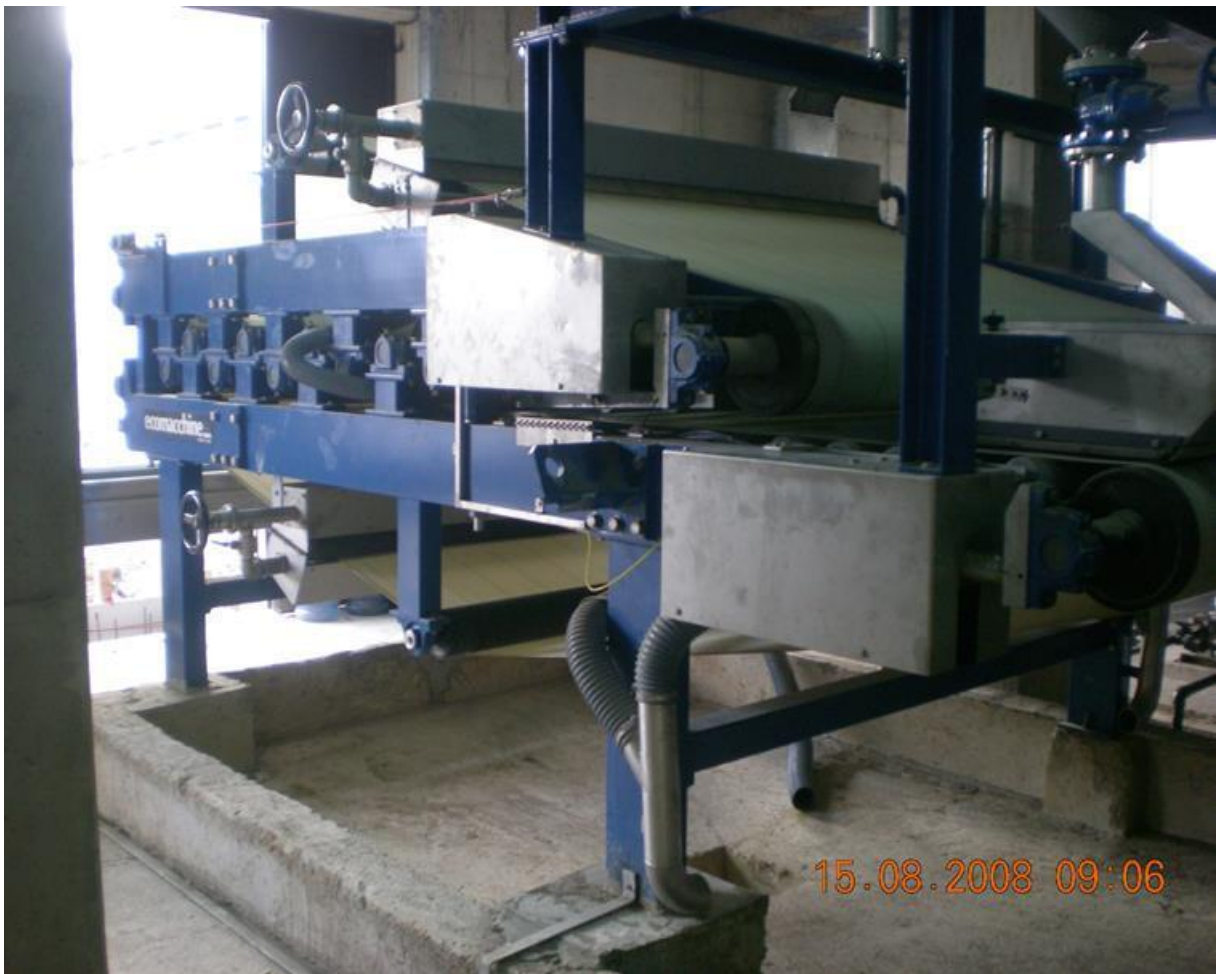
Sludge Belt Press General Appearance
