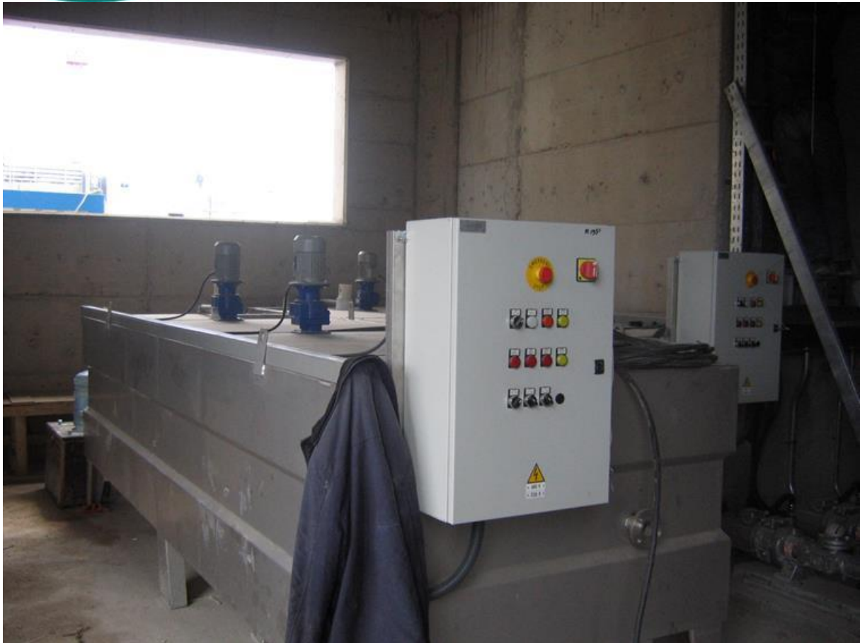
Polyelectrolyte Dosing Units
