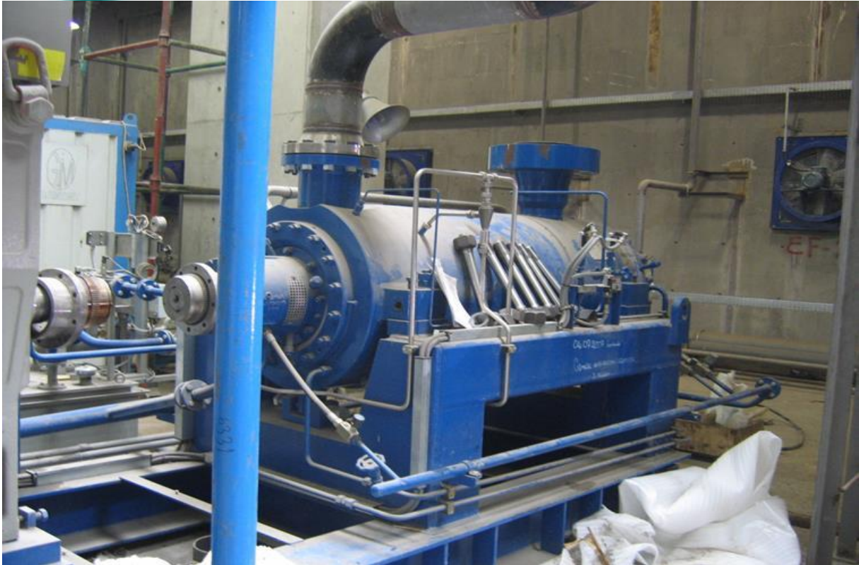
Descale Pump Genel Appearance
