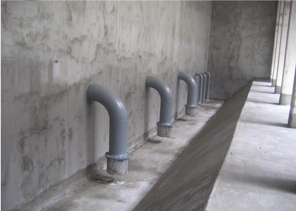
Pump Suction Pit and Strainer
