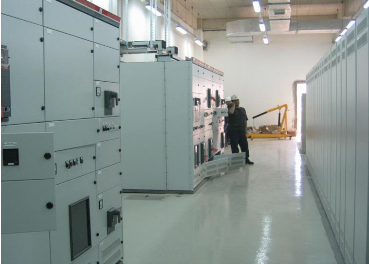
Electric Cabinet General Appearance
