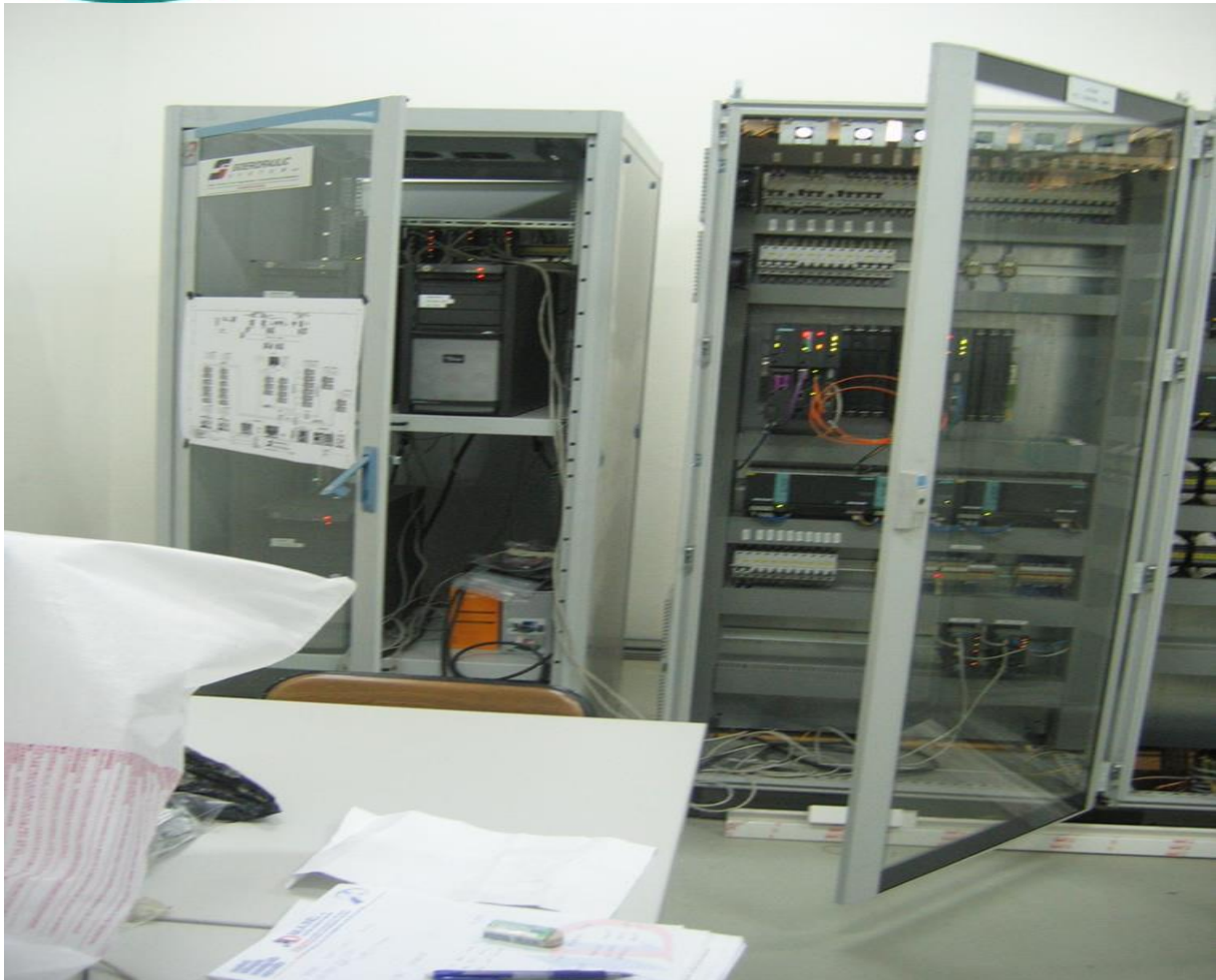
Operator Room and PLC System Cabinet
