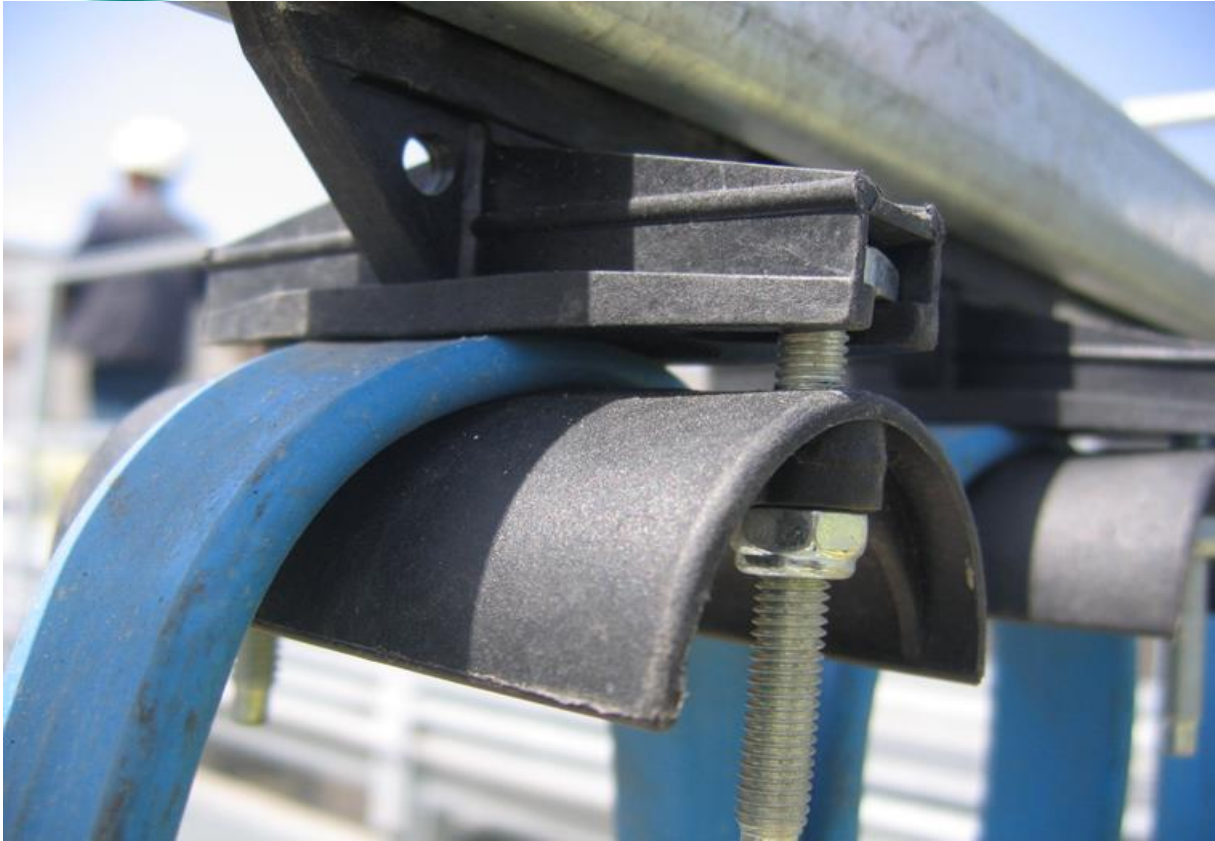
Settling Basin Scraper Bridge Cable
