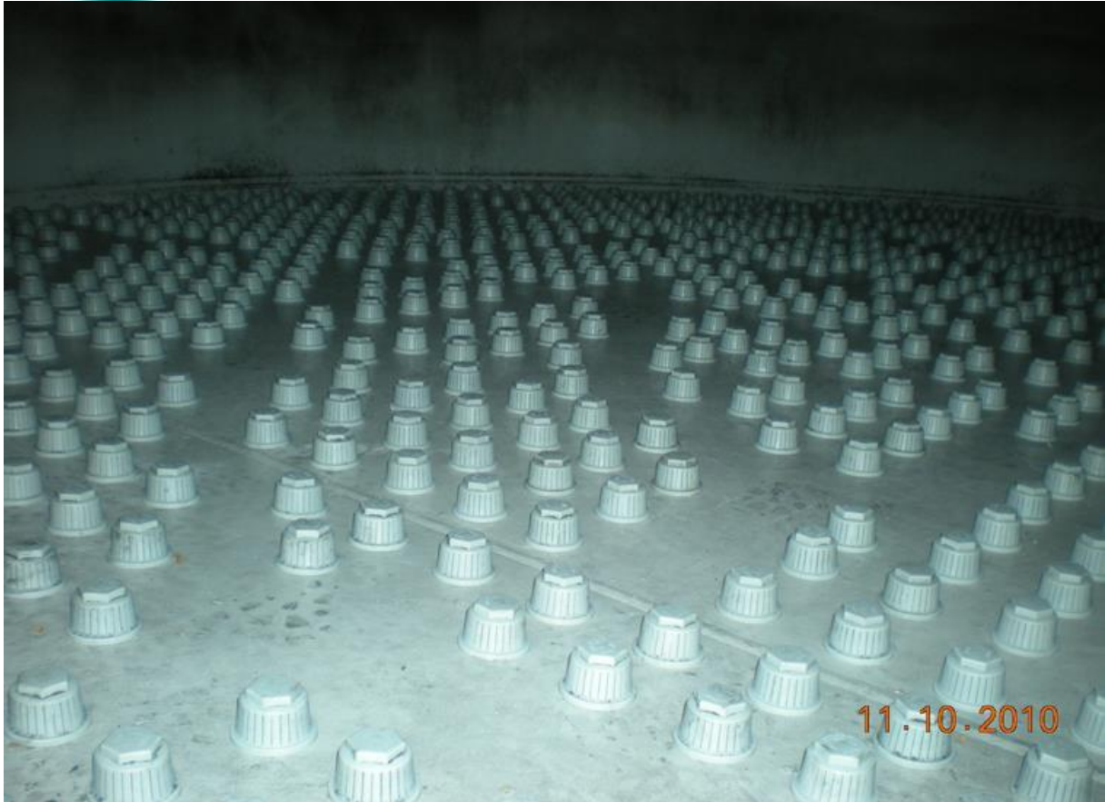
Sand Filter Inside (Nozzles Filters)
