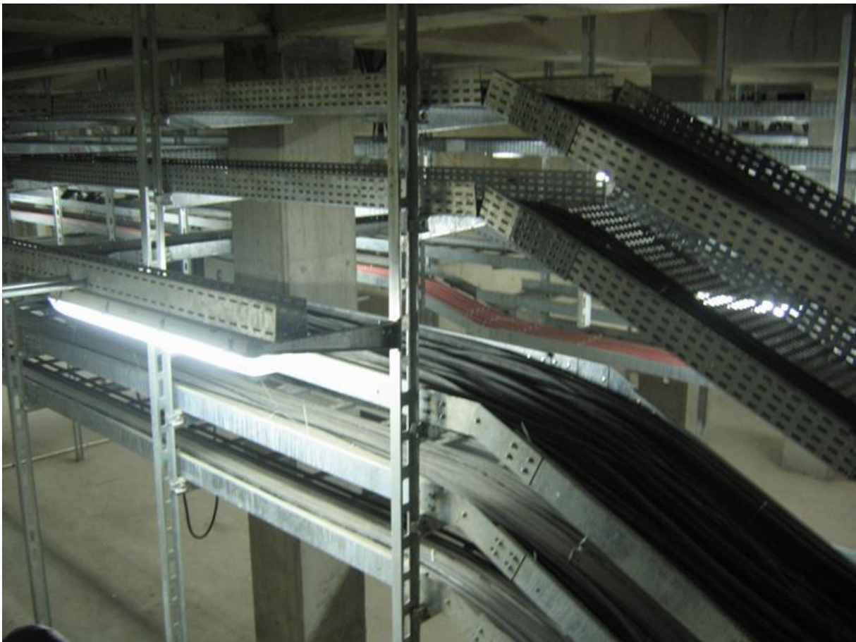
Cable Gallery General Appearance
