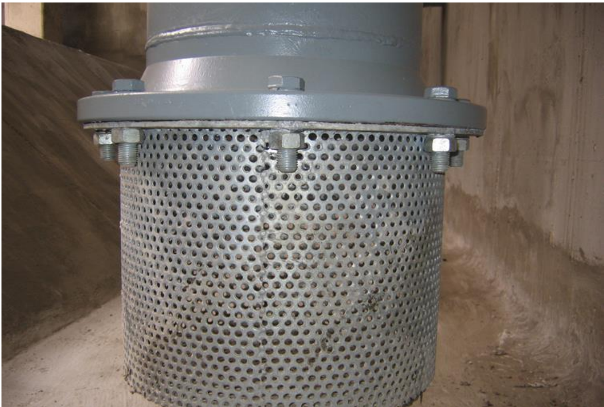
Pump Suction Pit and Strainer
