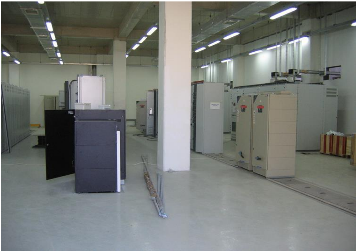
MCC PLC Cabinet General Appearance
