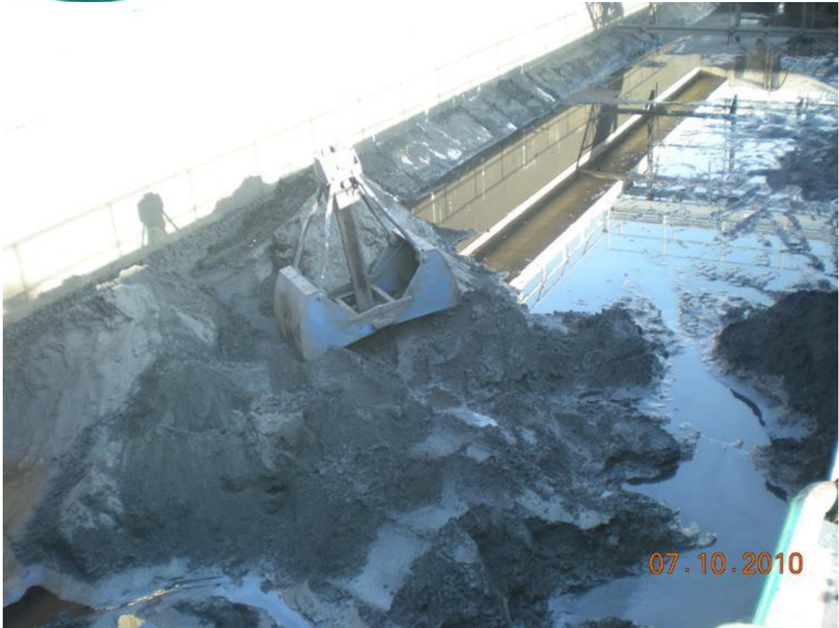
Settling Basin Bucket (Grab) and Hoist
