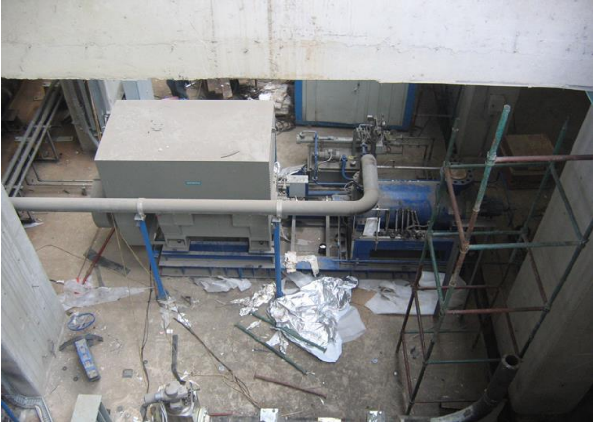
Descale Pumps Genel Appearance
