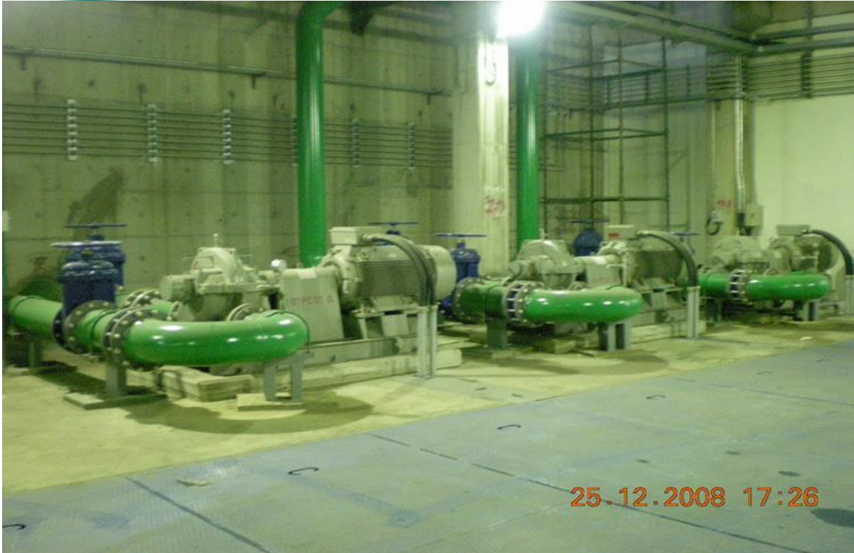
Indirect Circuit Pumps General Appearance
