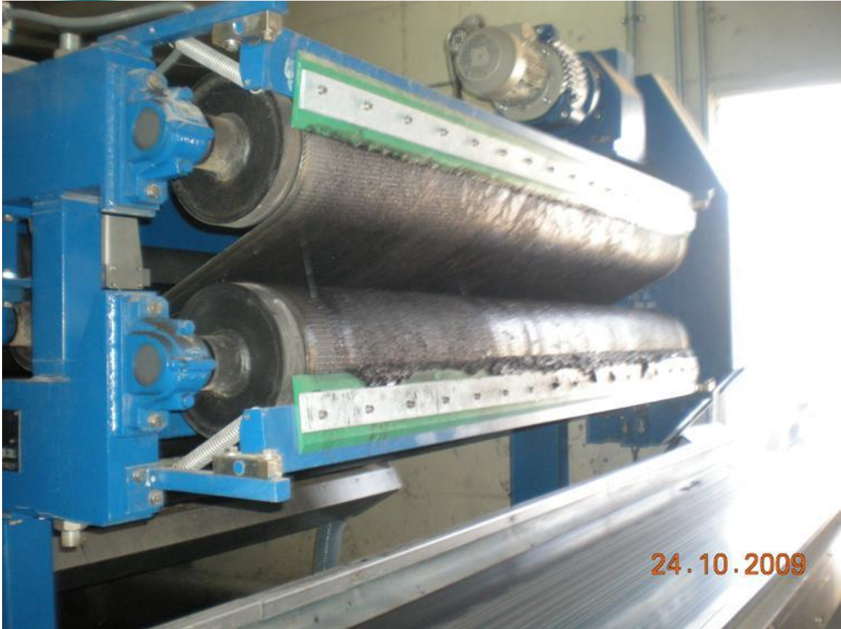
Sludge Belt Press General Appearance
