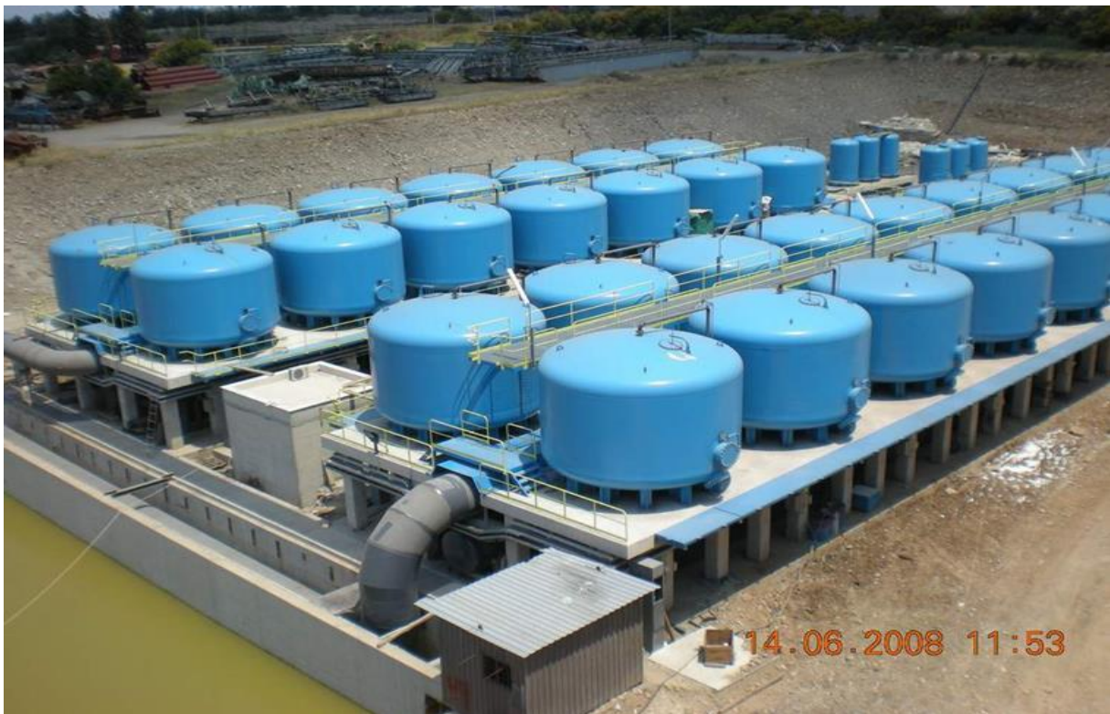
Sand Filter Area General Appearance
