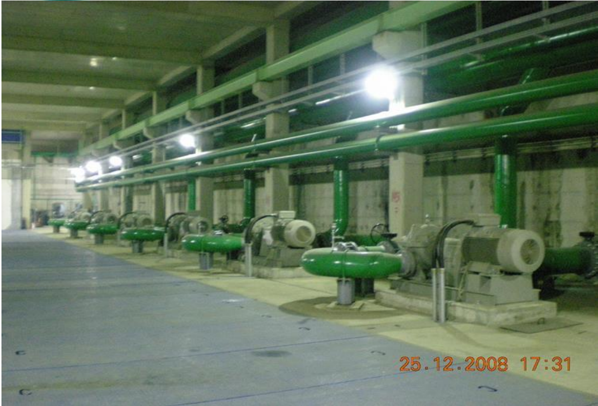
Direct Circuit C Pumps Genel Appearance
