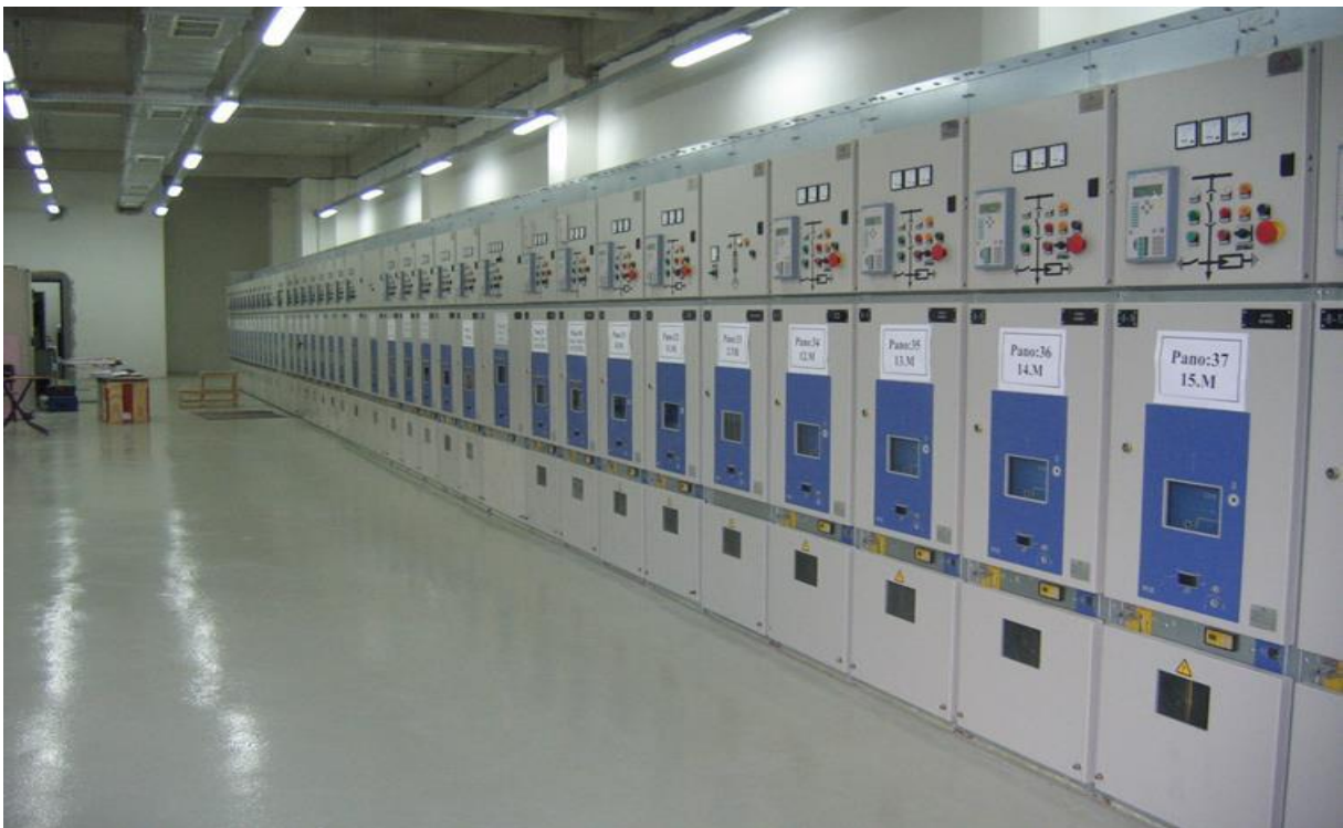
Electric Cabinet General Appearance
