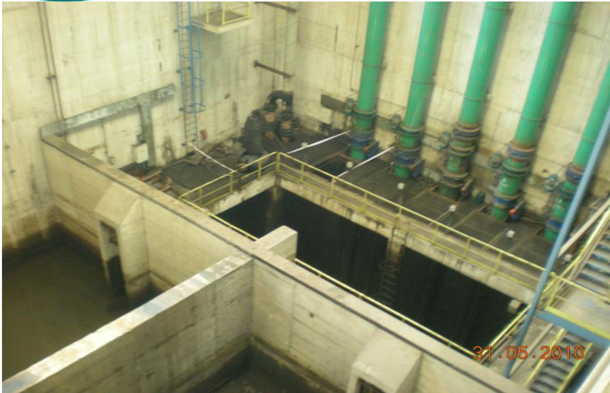
Scale Pit Submersible Pump Area
