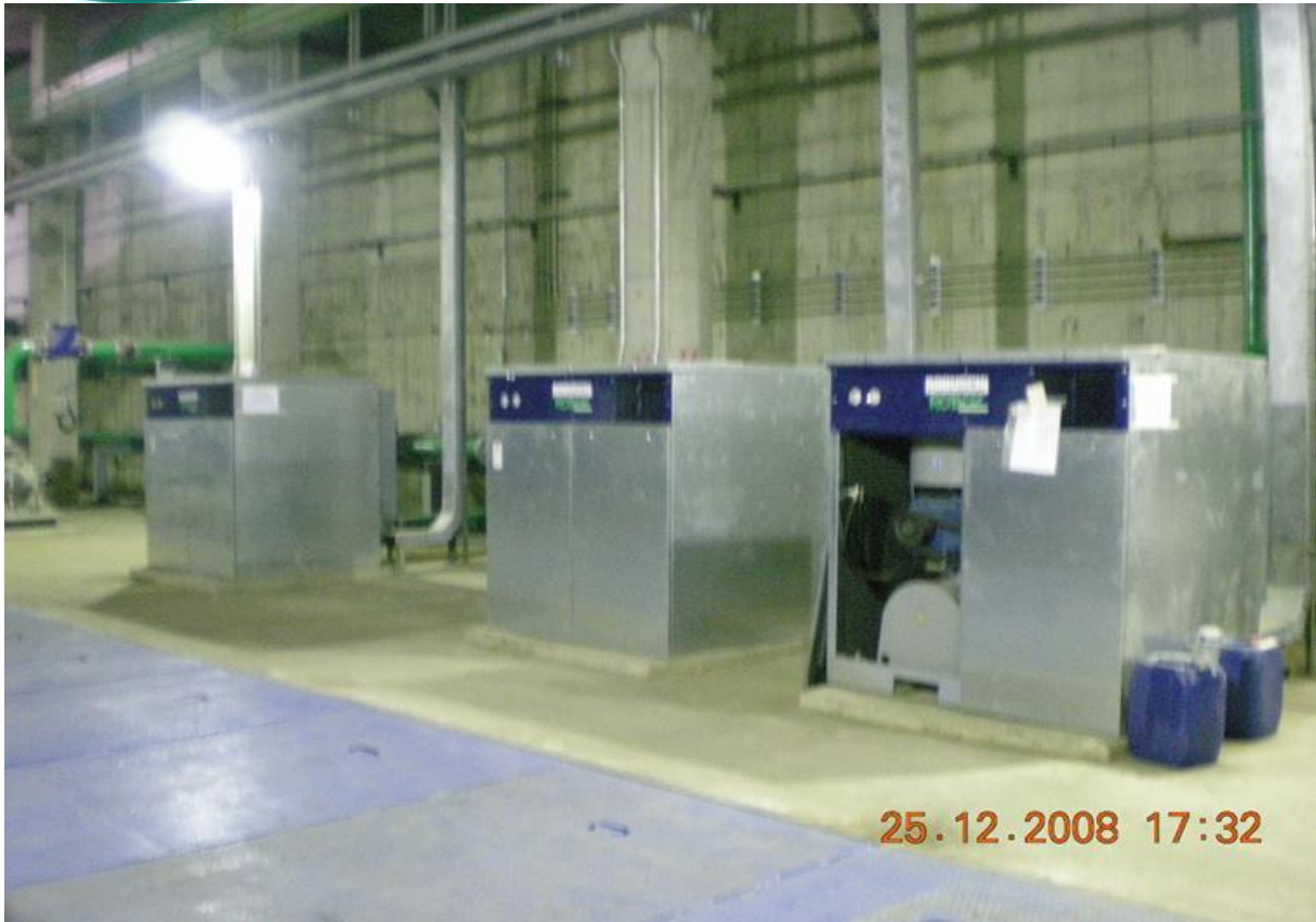
Sand Filter Blowers
