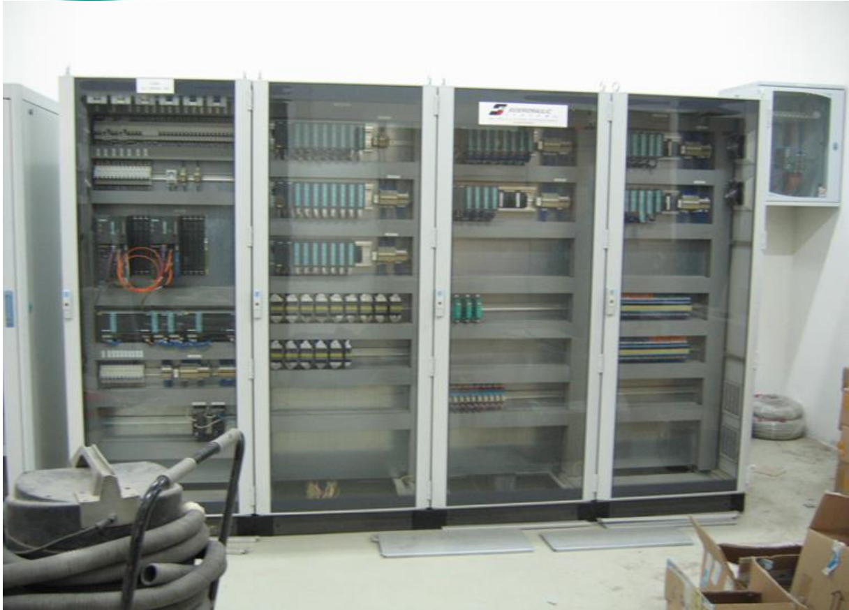
Operator Room and PLC System Cabinet
