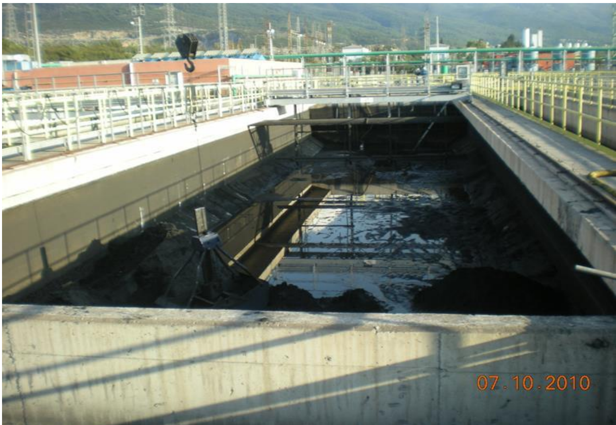
Settling Basin Bucket (Grab) and Hoist
