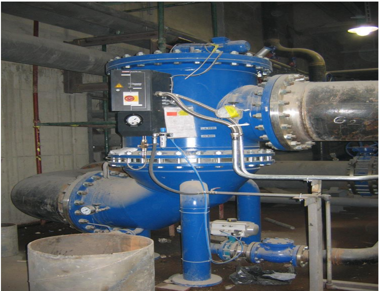
Descale Pump Suction Filters Genel Appearance
