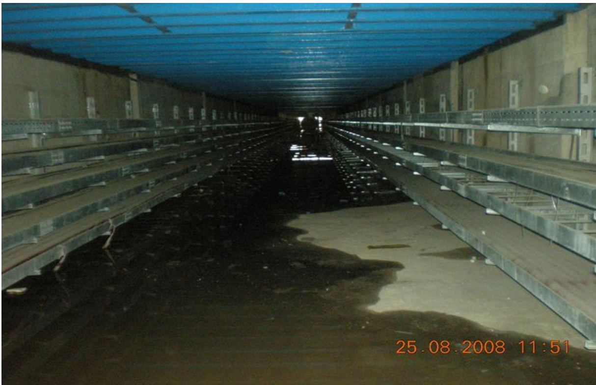
Cable Gallery General Appearance
