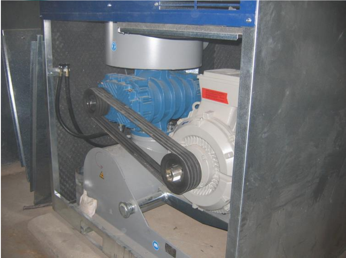
Sand Filter Blower Inside
