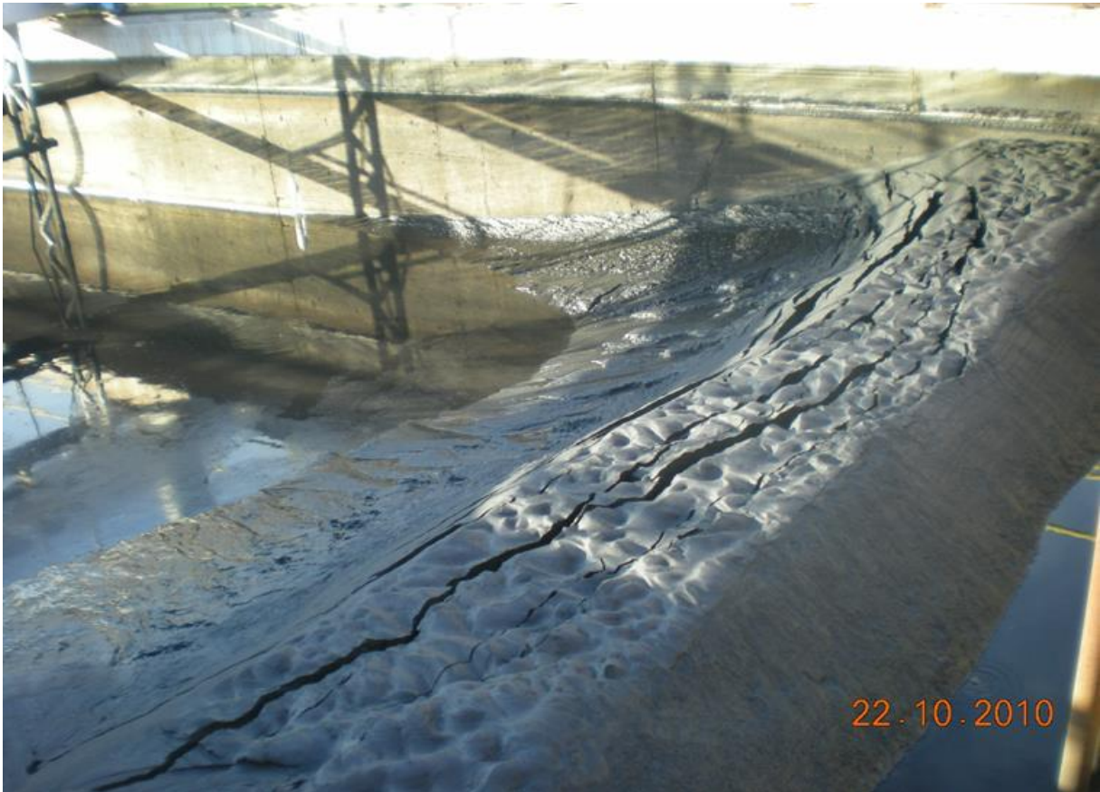
Settling Basin Sludge
