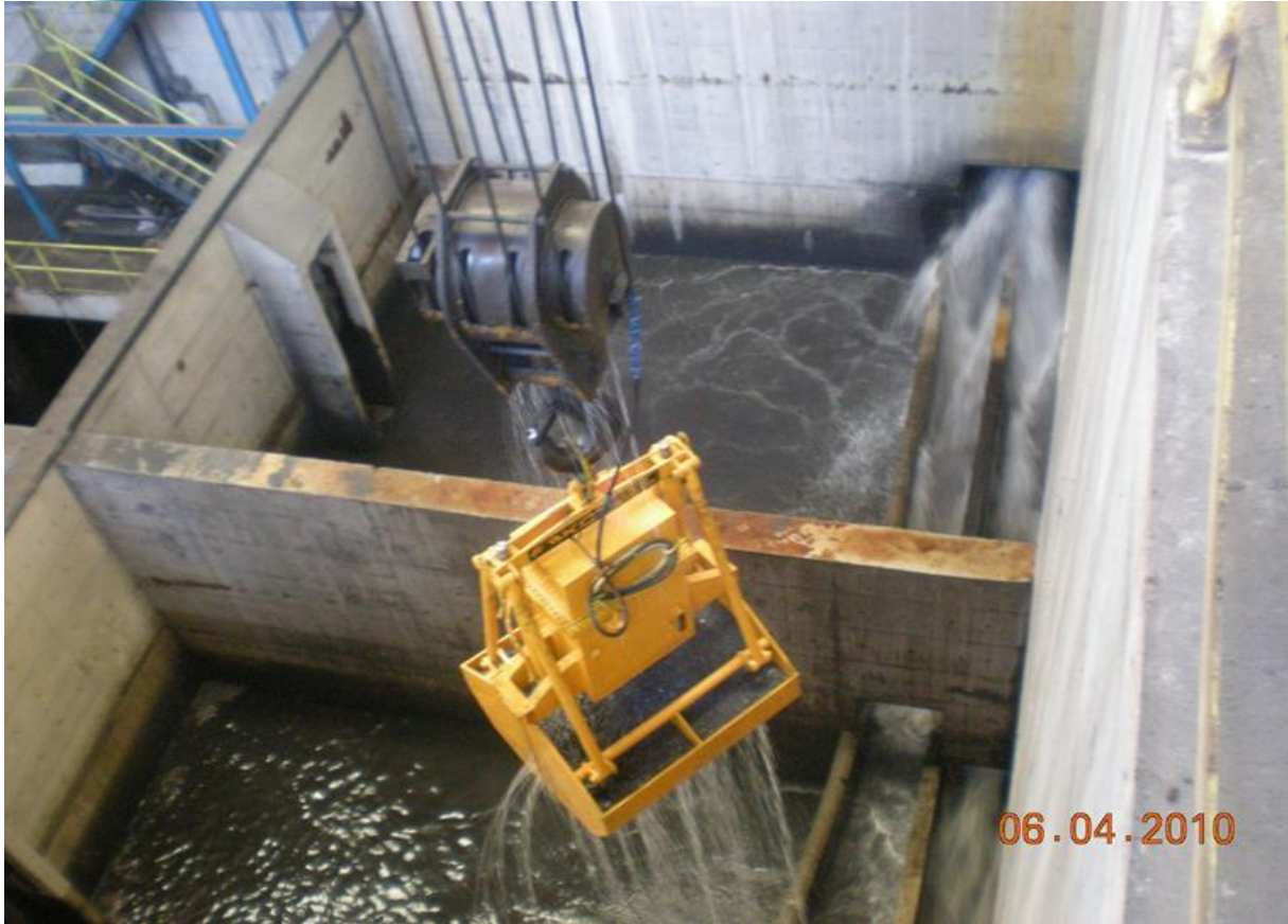
Scale Pit Bucket (Grab) and Hoist
