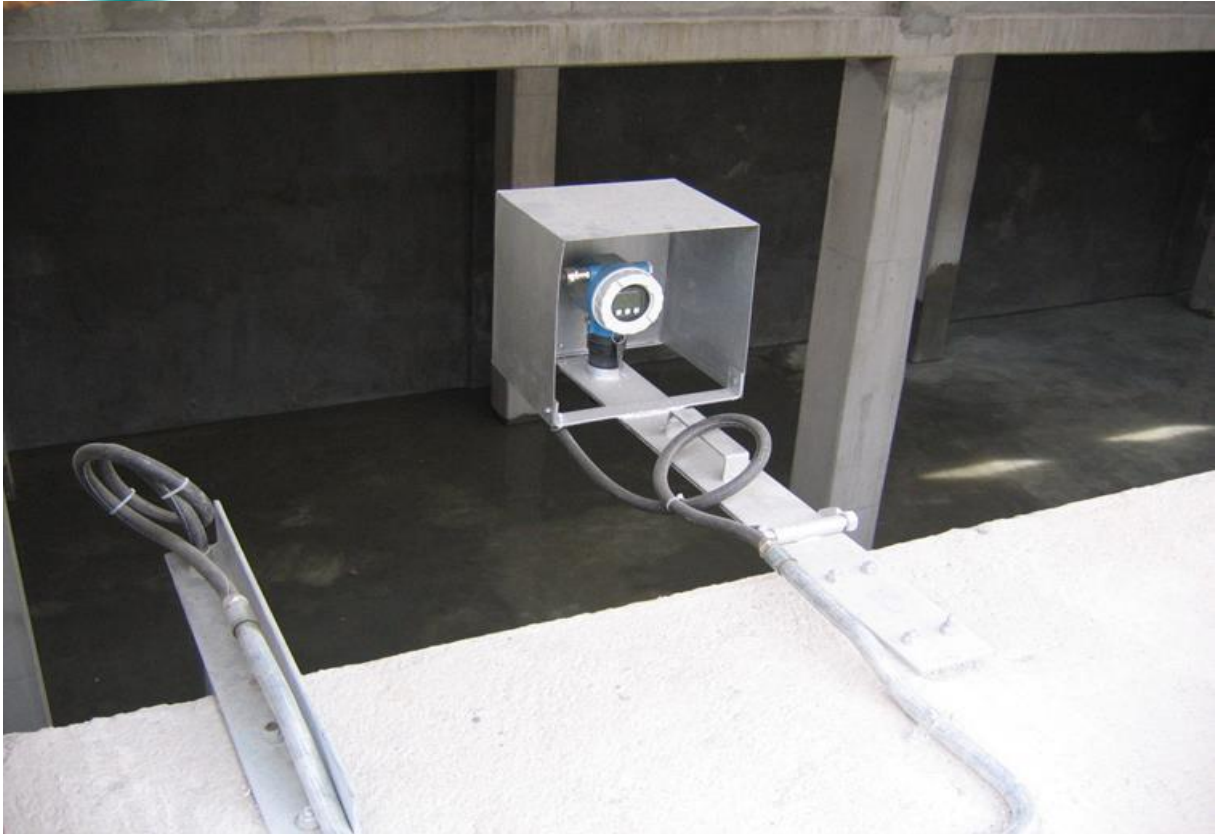
Cooling Towers Basin Level Transmitter
