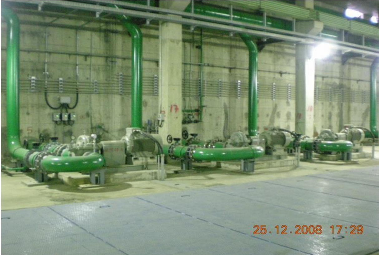
Direct Circuit B Pumps General Appearance
