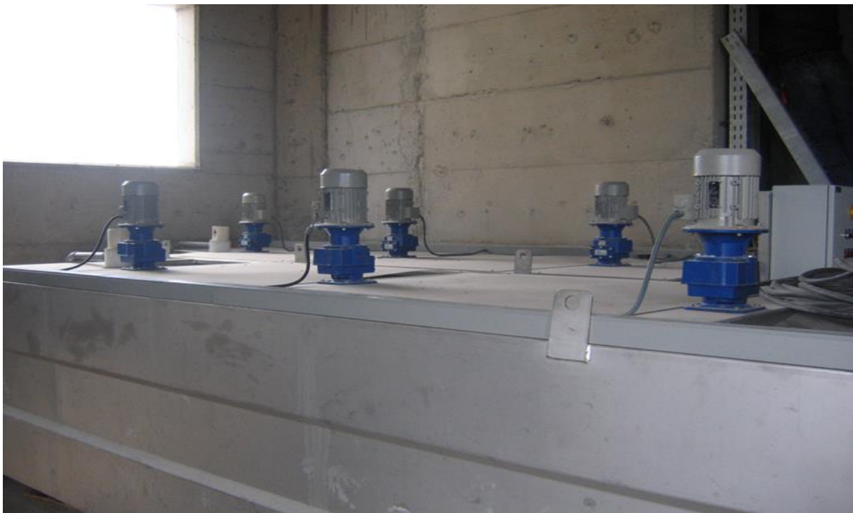
Polyelectrolyte Dosing Units
