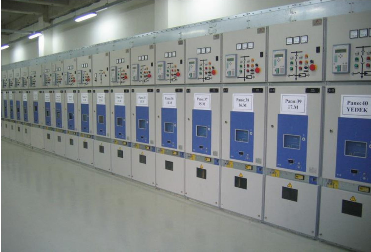
Electric Cabinet General Appearance
