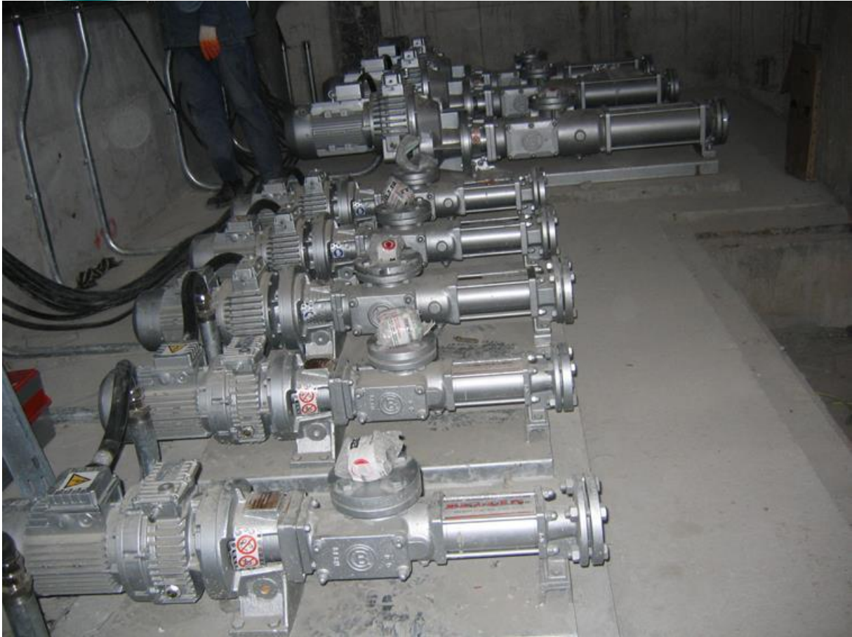
Sludge Pumps General Appearance
