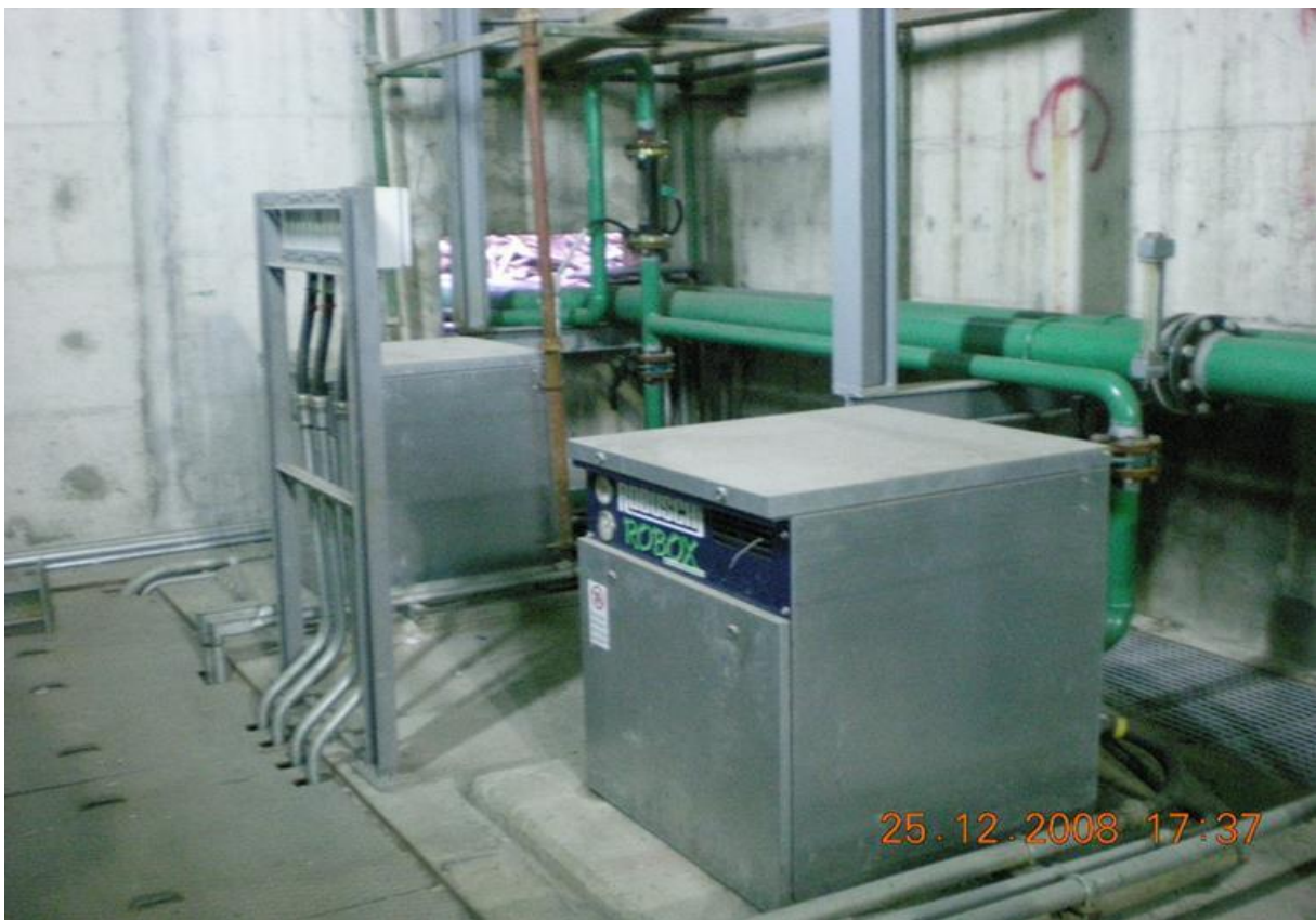
Sand Filter Blowers
