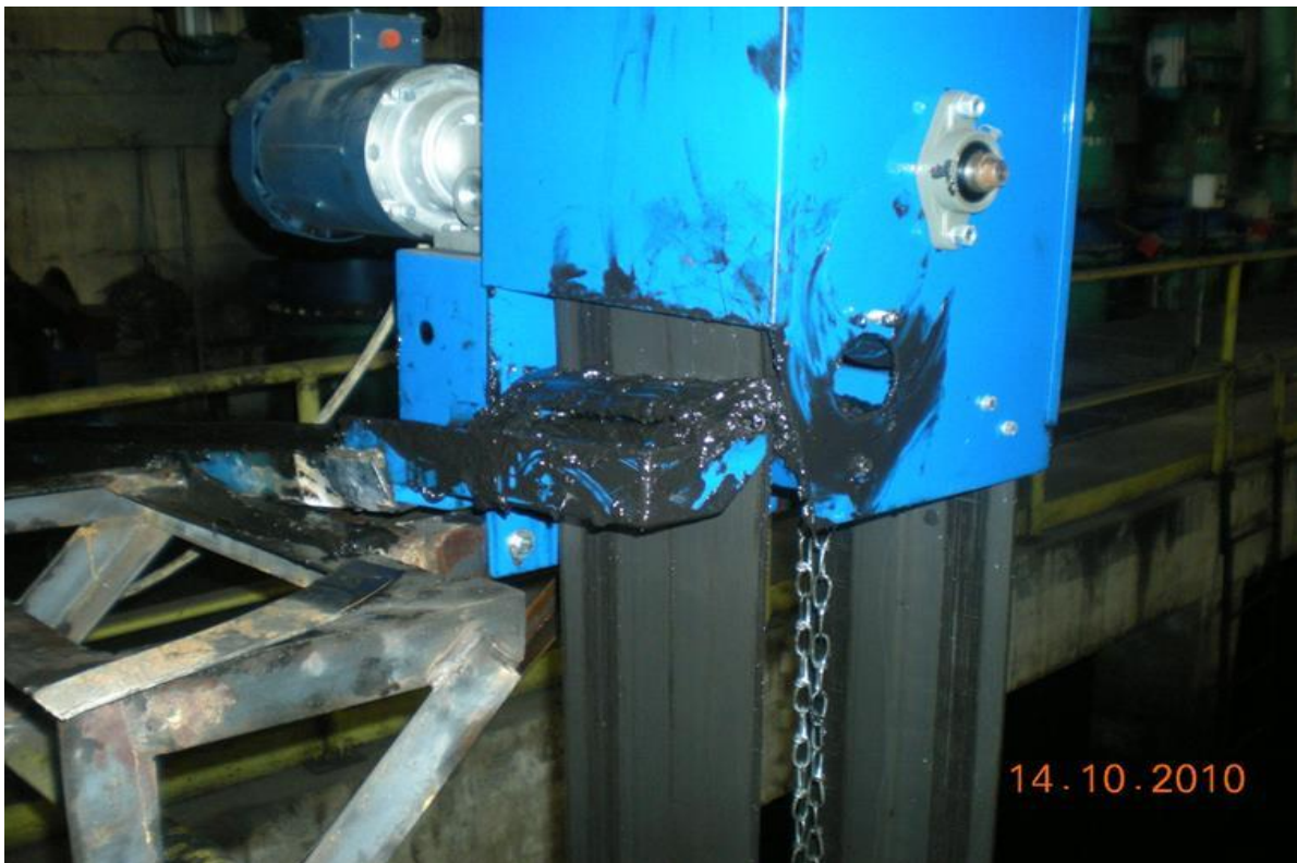
Settling Basin Oil Skimmer
