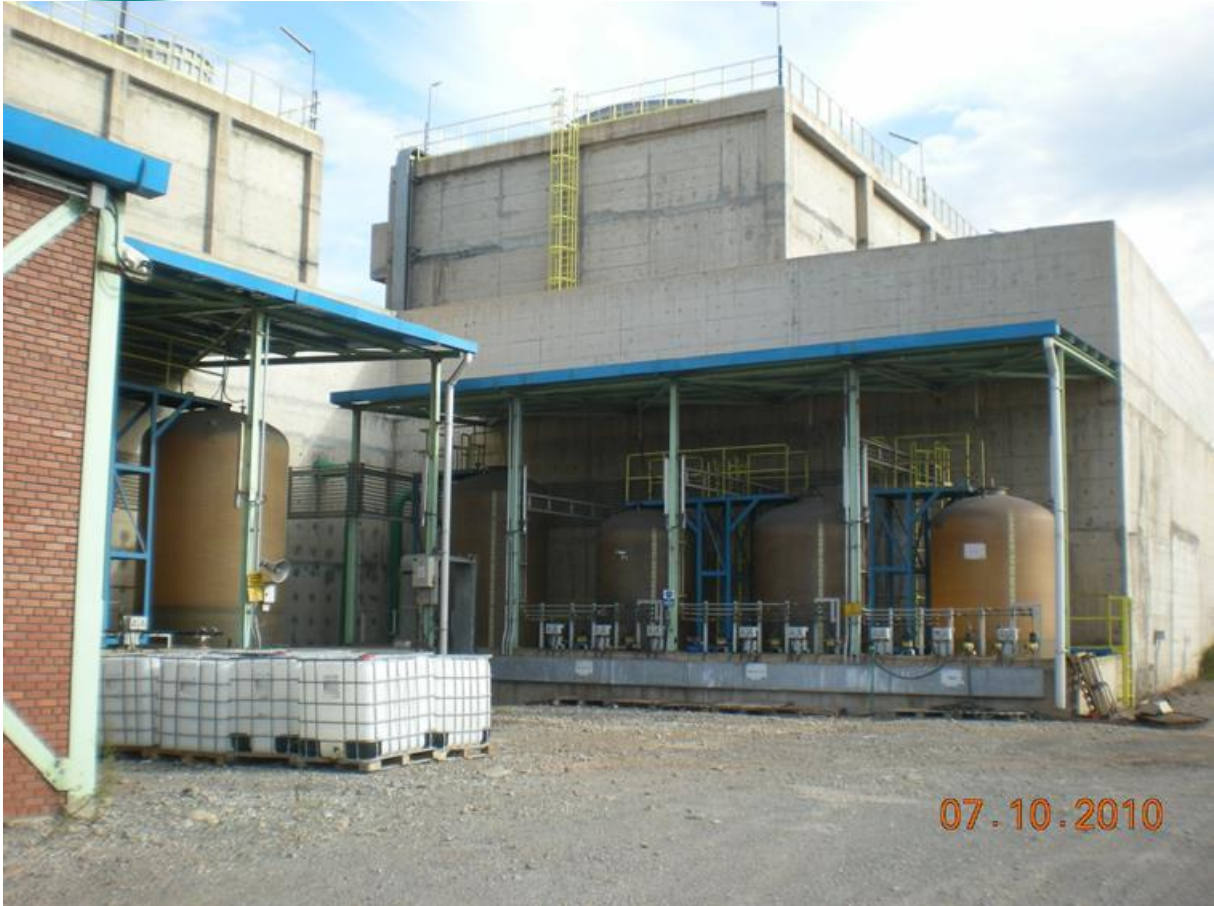
Chemical Dosing Units General Appearance
