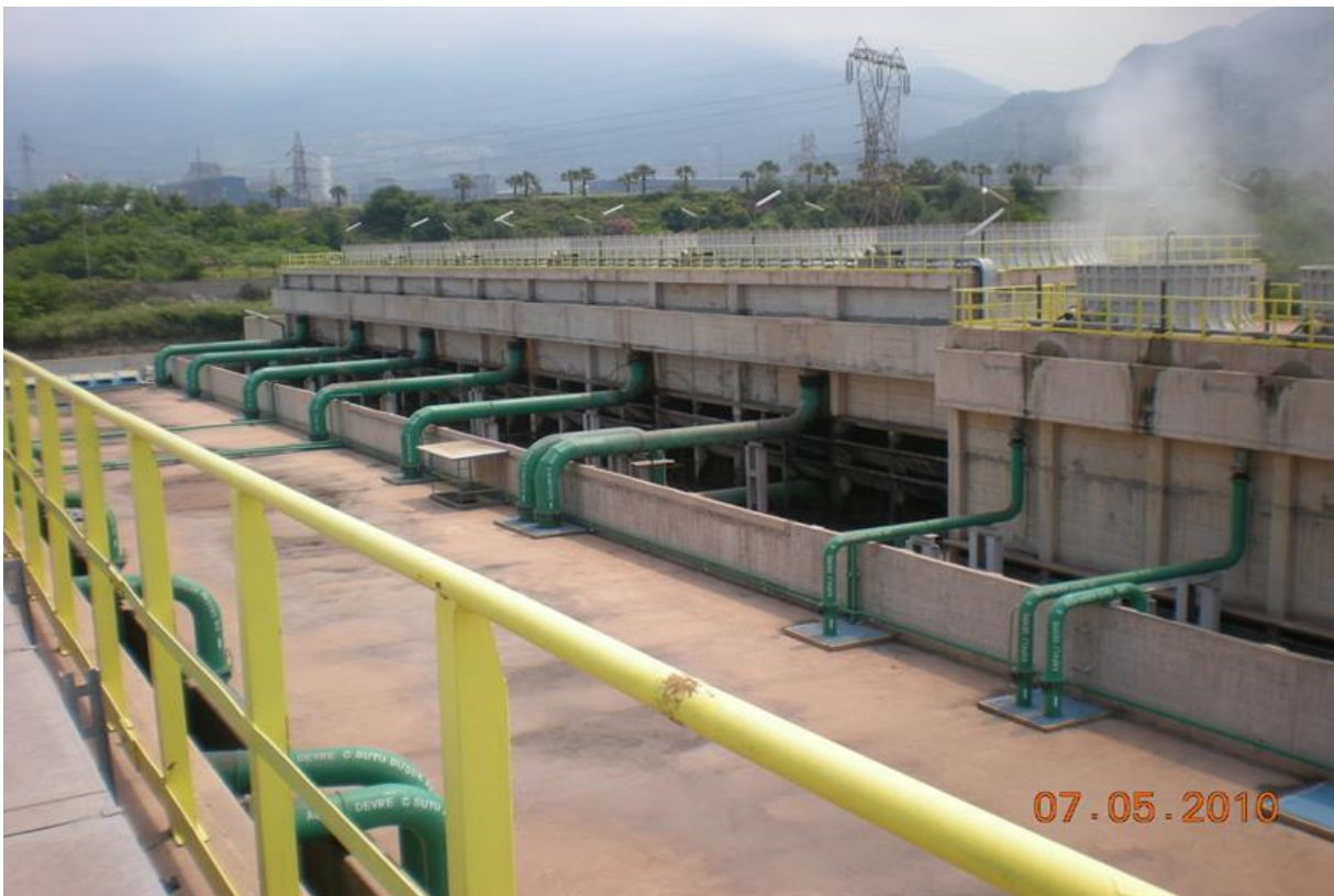
Cooling Towers General Appearance
